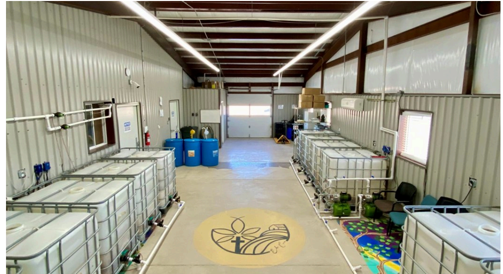
High-bay lobby — nutrient-tank plumbing, LED lighting, loading door
